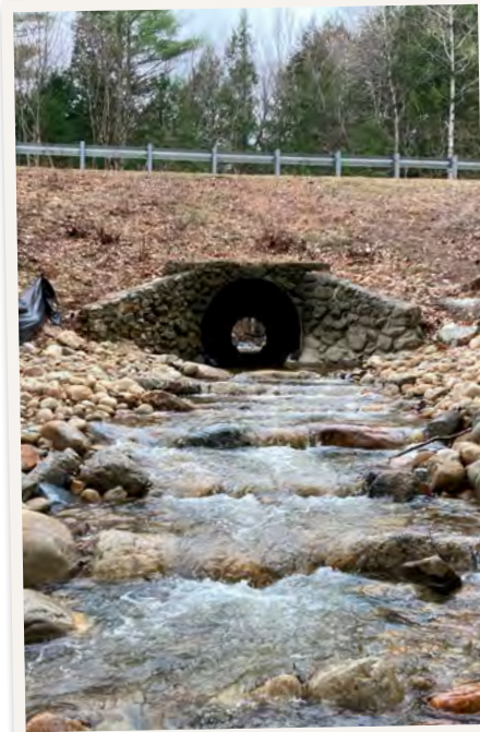
The Fish Habitat Program worked with NH Department of Transportation and UNH Civil Engineering to construct two fish ramps under Rt 89 in Warner to ensure that brook trout and other fish species can swim upstream through the two culverts.
